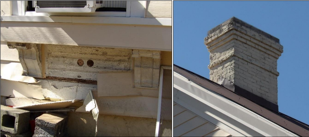
Photo 15: Detail of Scrolled Brackets and German Lap Siding on the Northeast Elevation (left); Detailed View of Easternmost Chimney (right).
